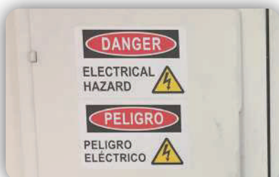
Electrical Panel Label
